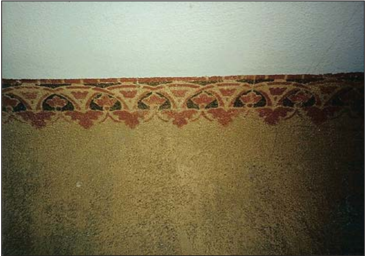
Detail view of finishes at ceiling of mezzanine prior to 1998 renovation. (Source: Gary Parks, 1998, http://www.flickr.com/photos/howardbhaas/285871917/ ).
