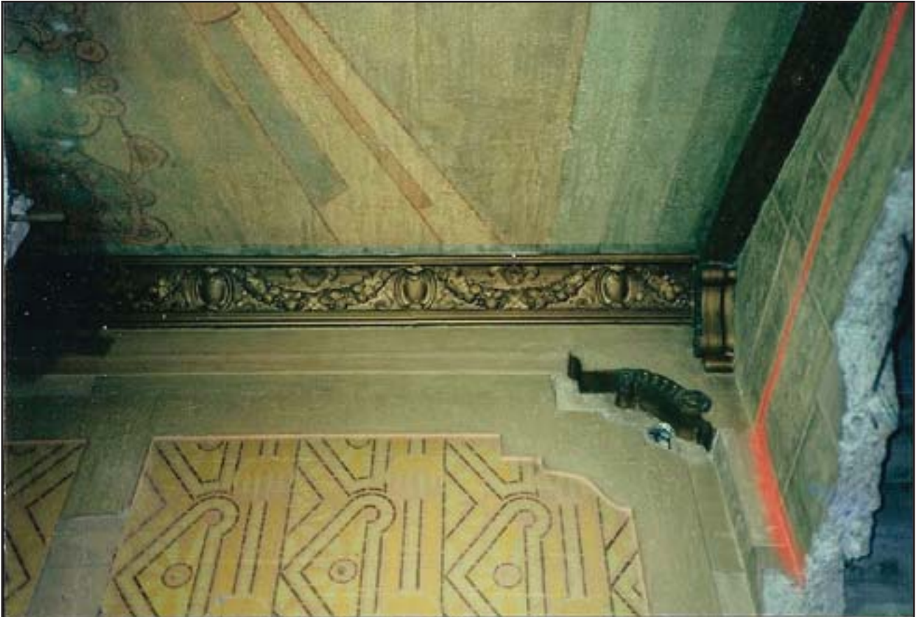
Detail of finishes at ceiling and wall of lobby prior to 1998 renovation. (Source: Gary Parks, 1998, http://www.flickr.com/photos/howardbhaas/285871917/ ).
