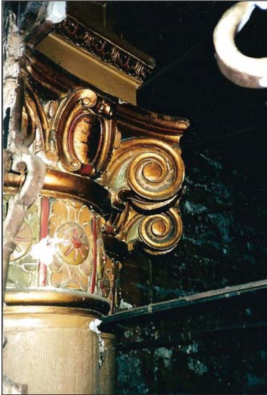
Detail view of capital in auditorium prior to 1998 renovation. (Source: Gary Parks, 1998, http://www.flickr.com/photos/howardbhaas/285871917/ ).
